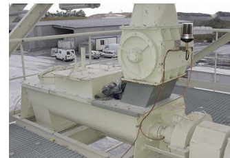
Mineral industry: lime factory: lubrication of 4 screw drive bearings.
