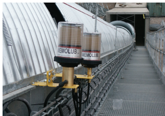
Mineral industry: lubrication of conveyor belt bearings.
